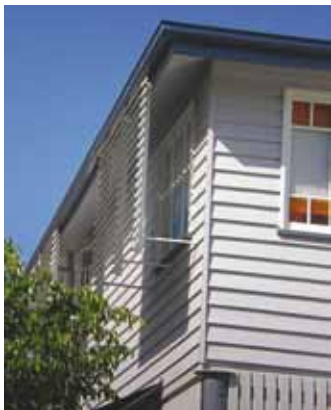
Figure 9 An example of how effectively the vertical screen shades the window from low-angled sun.
